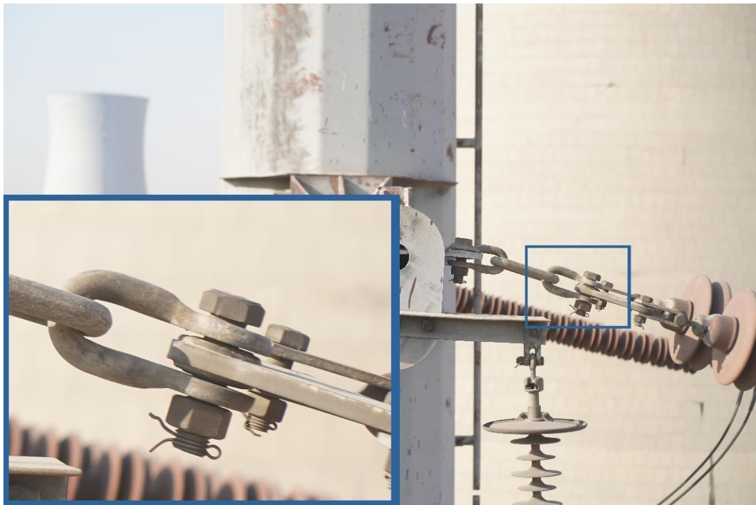
Transmission Line Against the light at 5m
